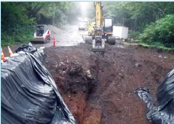
The top of the 12' diameter tree stump in the middle of the excavation
