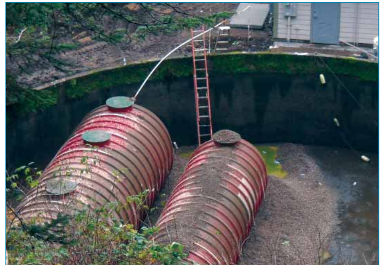
The aeration basin after being pumped out and the first tanks installed
