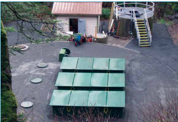
The aeration basin after it was covered and the treatment pods installed
