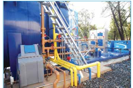
Chemical feed and associated piping for MBR
