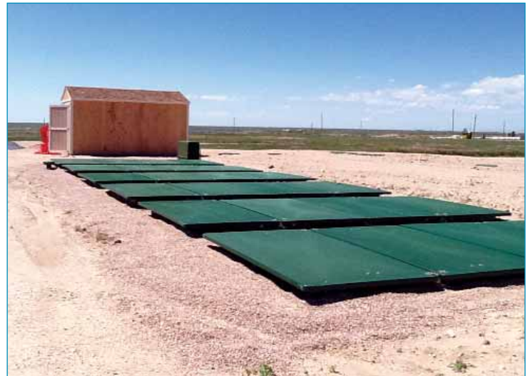
A view of the completed treatment system showing the tops of the AdvanTex Pods
