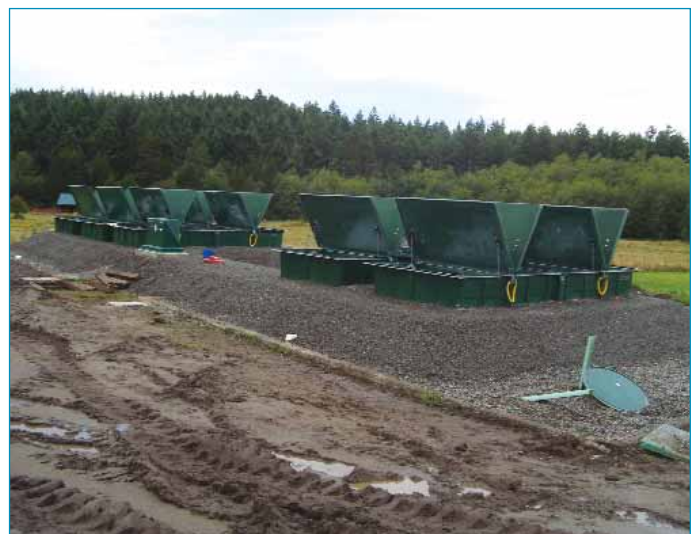
Advantex pods installed on top of existing sand filter
