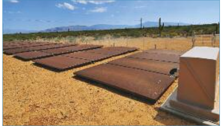
A view of the installed Orenco Advantex treatment pods
