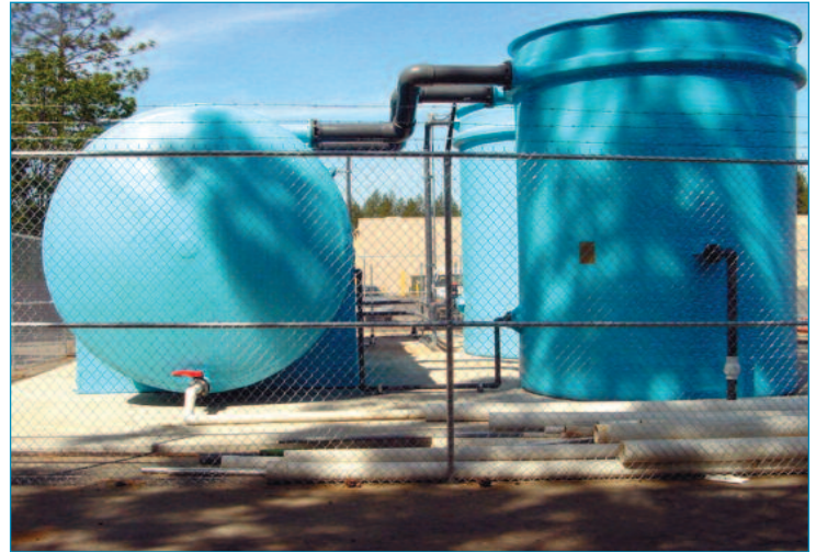
IWS installed the modified SBR as part of the new treatment system
