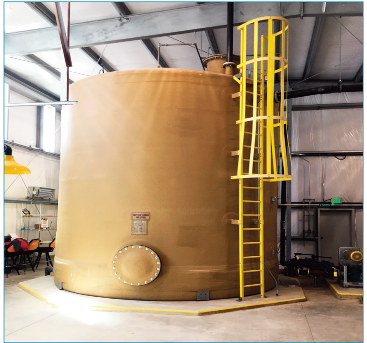
Flow equalization tank (21,000 gallons)
