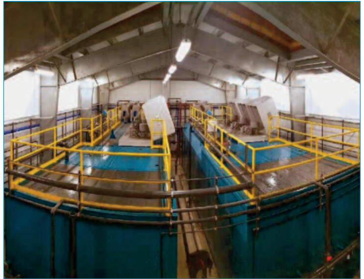
MBR Treatment System in Building
