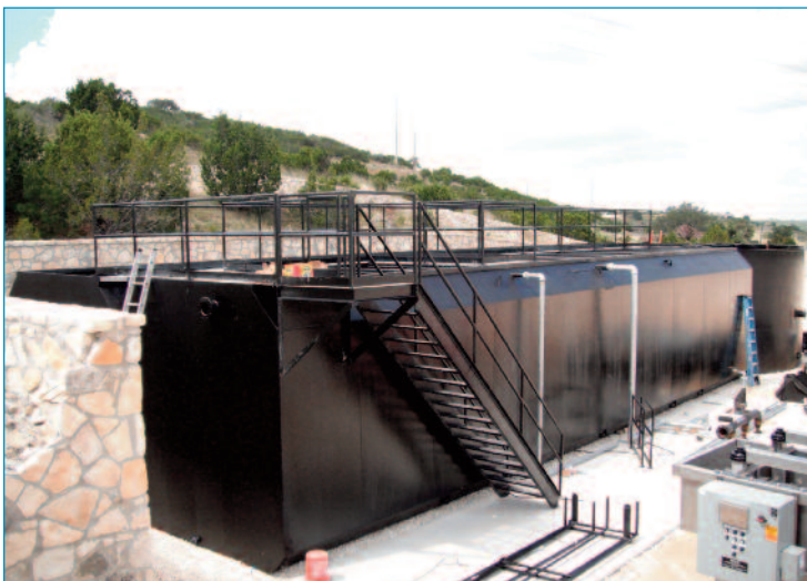
Treatment tank in place
