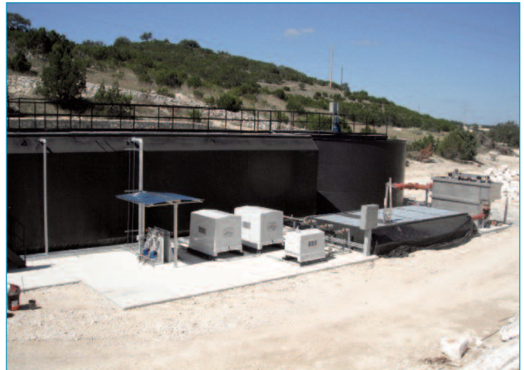
Blowers in foreground of treatment system
