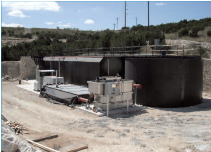
Completed System View
