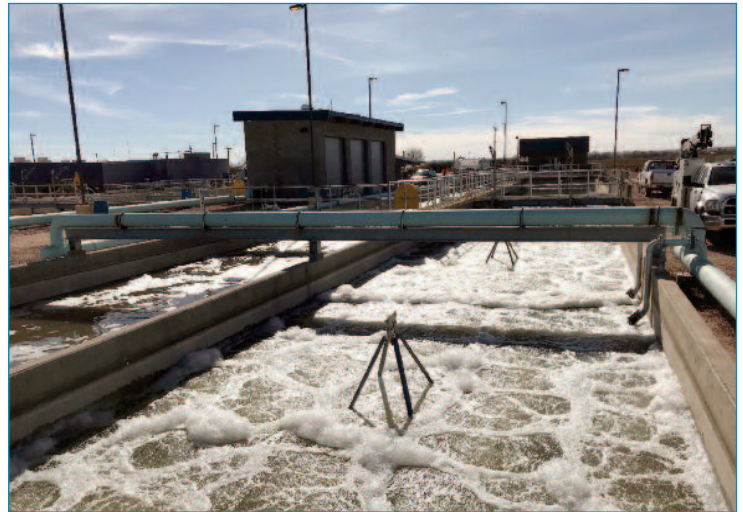
Effluent flowing in Oxidation Ditch
