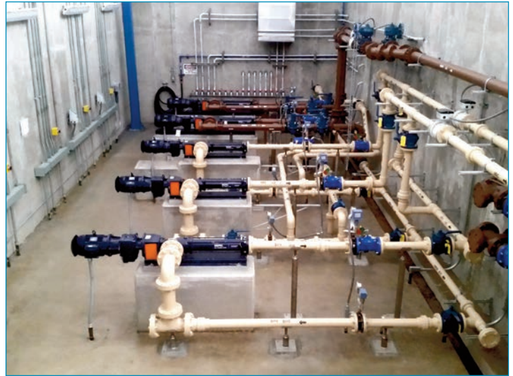
Process Piping Adjacent to Treatment Basin
