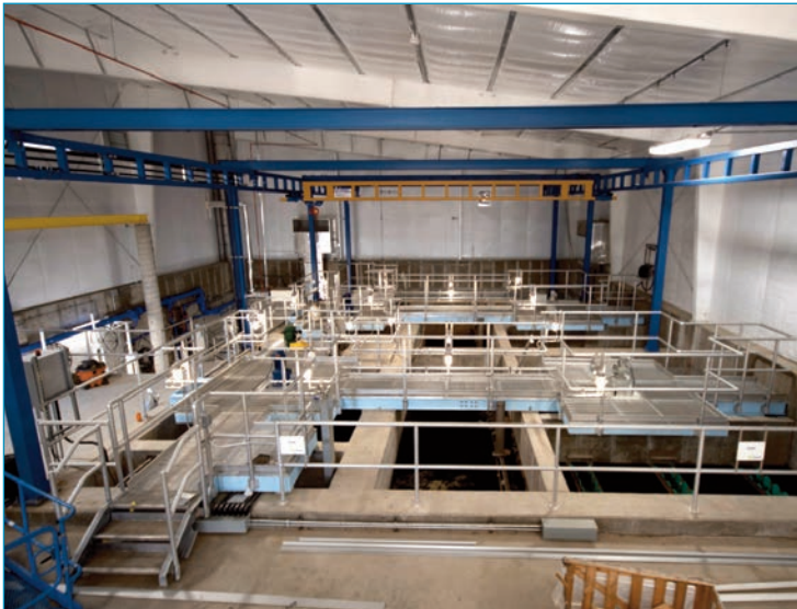
Process Treatment Basin
