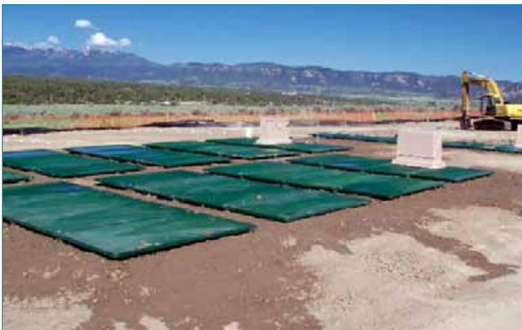
The completed treatment system
