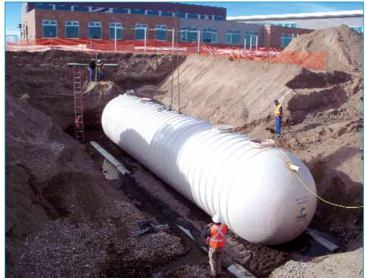
The 30,000 gallon Containment Solutions Tank
