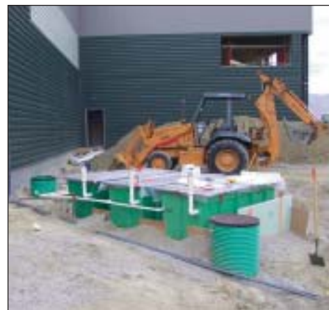
AX-20 Units and Tank Risers
