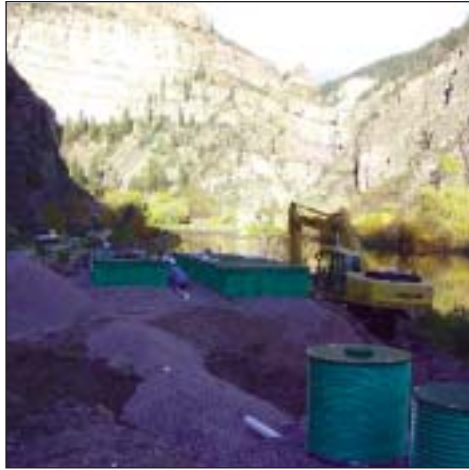
Tank and Treatment Area at Hanging Lake
