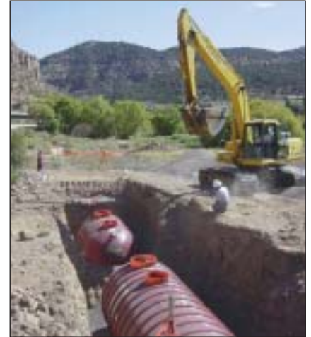
Septic and Recirculation Tank at Bair Ranch
