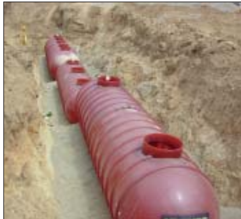
Septic, Recirculation, and Dosing Tanks
