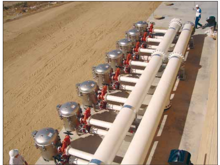
Pre-filters and Influent Manifold Assemblies
