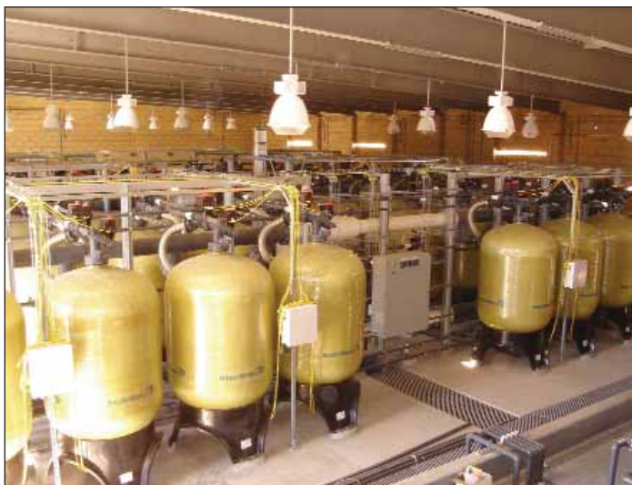
Completed Ion Exchange Treatment Trains
